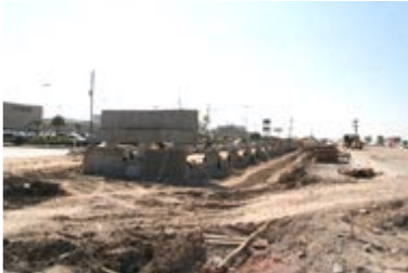
Construction of the retaining wall of the new I-10 eastbound entrance ramp west of Bunker Hill
