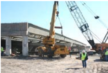
Erection of steel beams for the I-10 eastbound mainlanes overpass at Gessner
